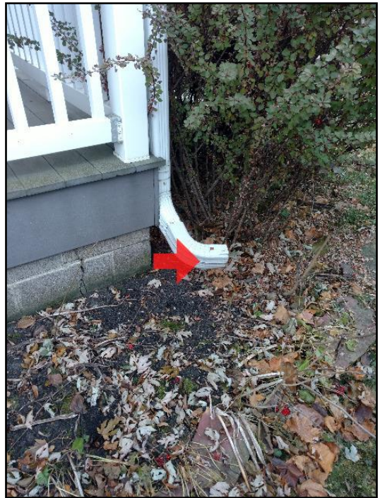
Should discharge 6 feet from building
