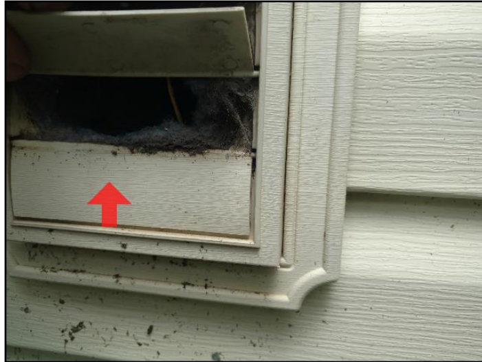
Plugged dryer vent
