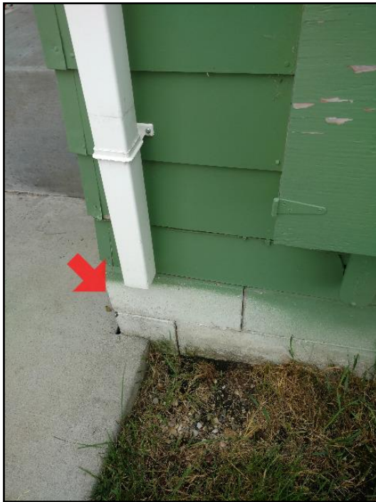
Should discharge 6 feet from building
